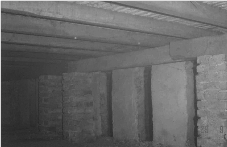
Fig. 6. The under-plenum duct inside the drying bin of an 8 t dryer (“Ong gio chim” in Vietnamese).
