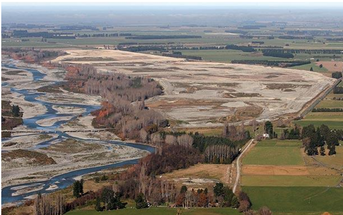
Figure 1: Off river storage adjacent the Rangitata River under construction (Source: Timaru Herald)
