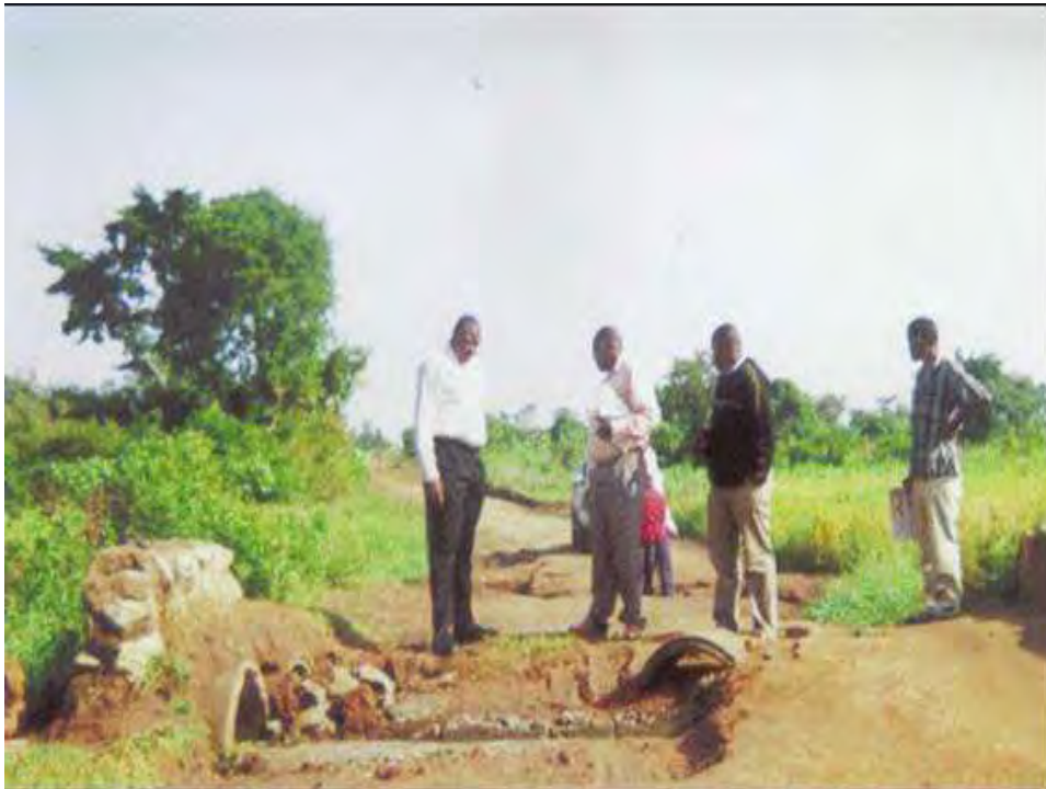
Figure 4: Broken culverts along Opedura-Akisimu road, Angule Sub-county, Pallisa District
