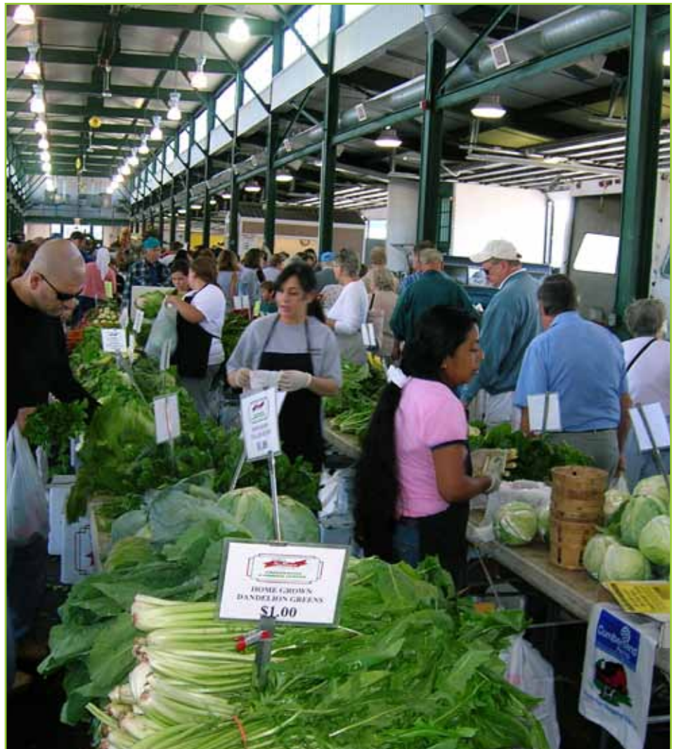
Central New York Regional Market has replaced these HID lights (shown) in their market sheds with more energy efficient LED lights.
