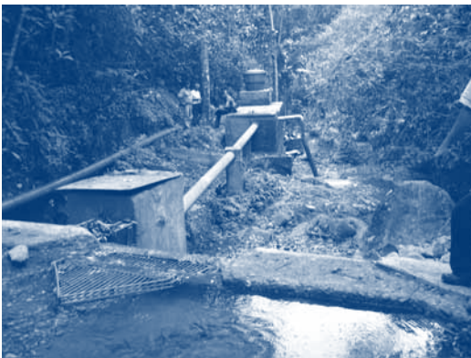
Figure 3.22. A multiplicity of pipes makes it difficult to monitor water intakes in the stream of the El Chocho catchment (photo: Grupo GIRH - Cinara)
