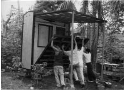
c. The floor is unfolded from the vertical to the horizontal position, mounted on prefabricated footings and levelled
