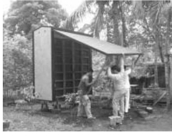
b. The roof, which is an integral face of the casing, is raised and temporarily supported
