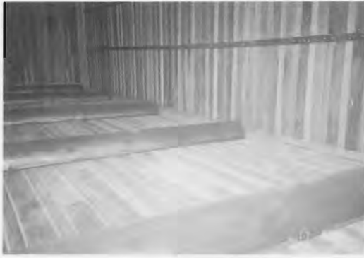
Figure 1. Air ducts in elevated wooden shed.
