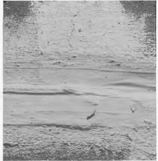
Fig. 23. Joint sealing (upper) and crack sealing (lower), typical applications of bandage seals.
