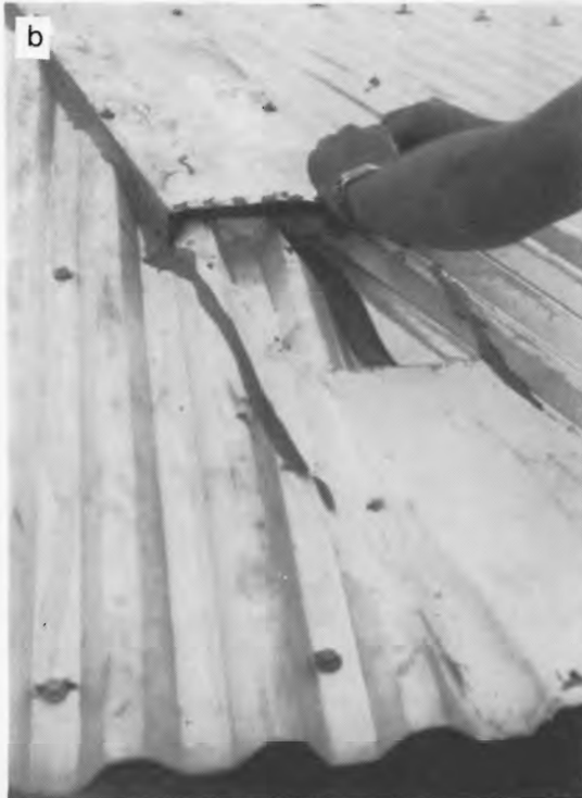
Fig. 11. (a) Location of a potential gas leakage path along sheeting laps. (b) Sealing under ridge capping. Note that sides of capping are sealed with silicone.
