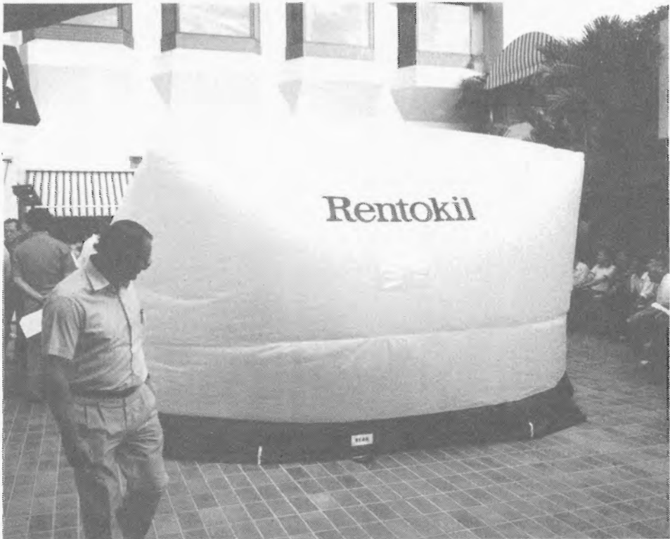
Fig. 1. Sealed enclosure of Rentokil Fumigation System
