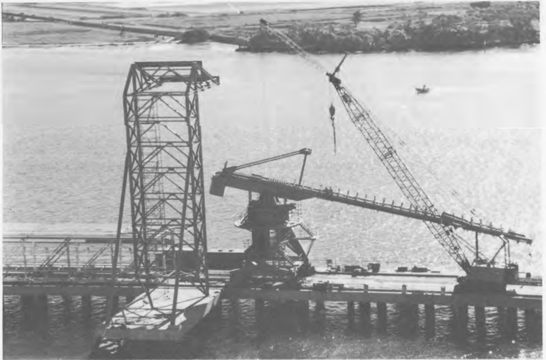
Fig. 4. Shiploader at Fisherman Islands grain export terminal, Brisbane, Queensland, Australia: photograph taken during construction in 1985
