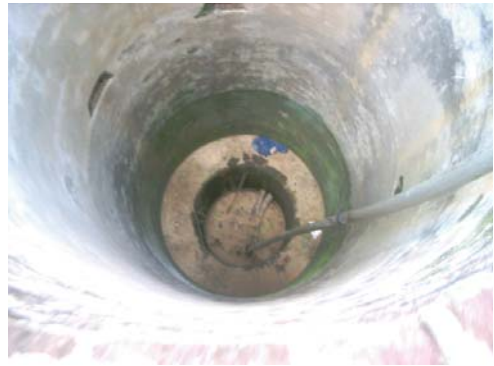
Aspect of the dried well and dropped tubewell instrument to the bottom.
