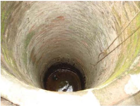
Lowering of water level of surface wells due to excessive sand mining in the area.
