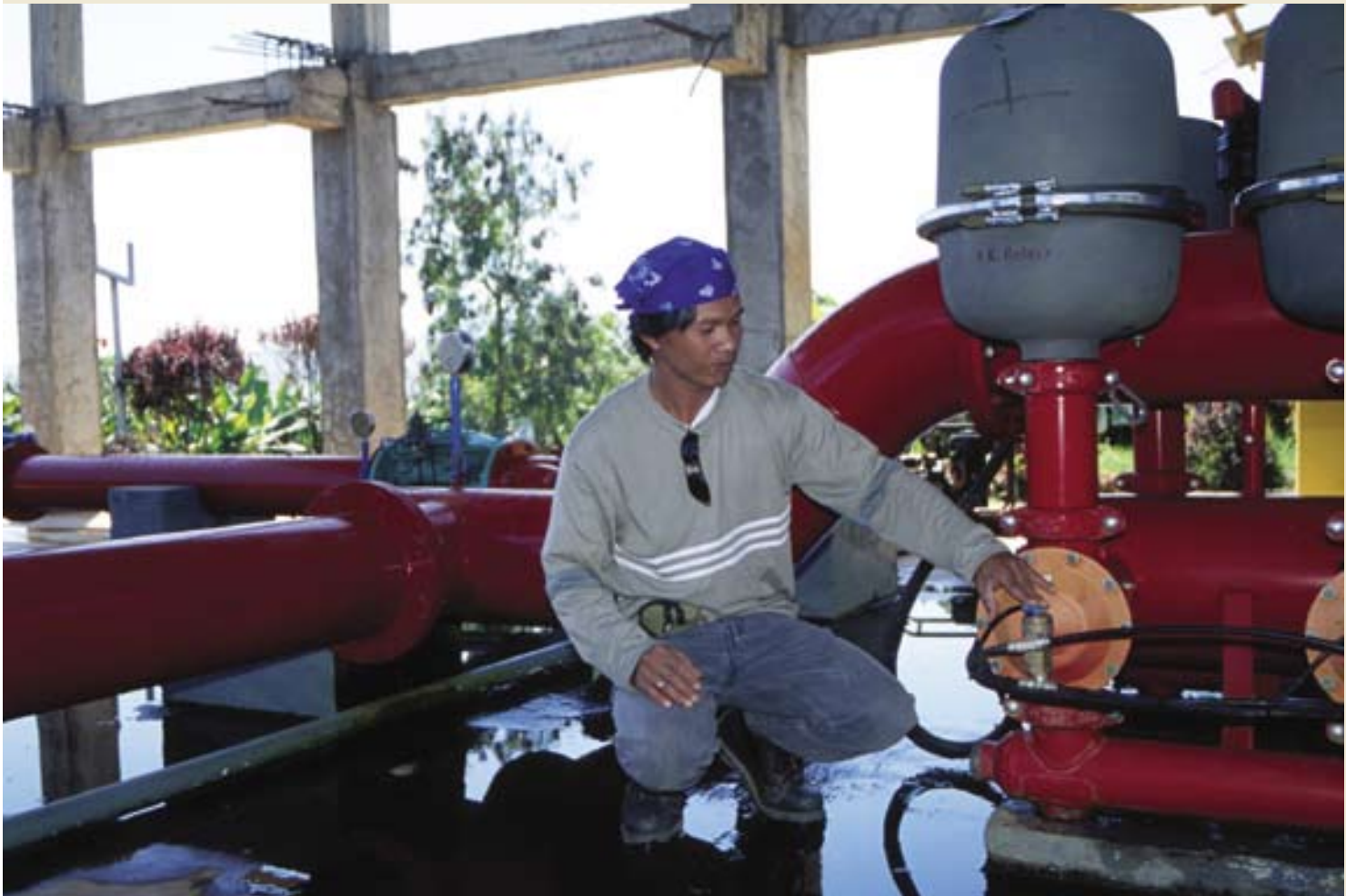
A worker at MKAVI checks the plantation's irrigation control system.
