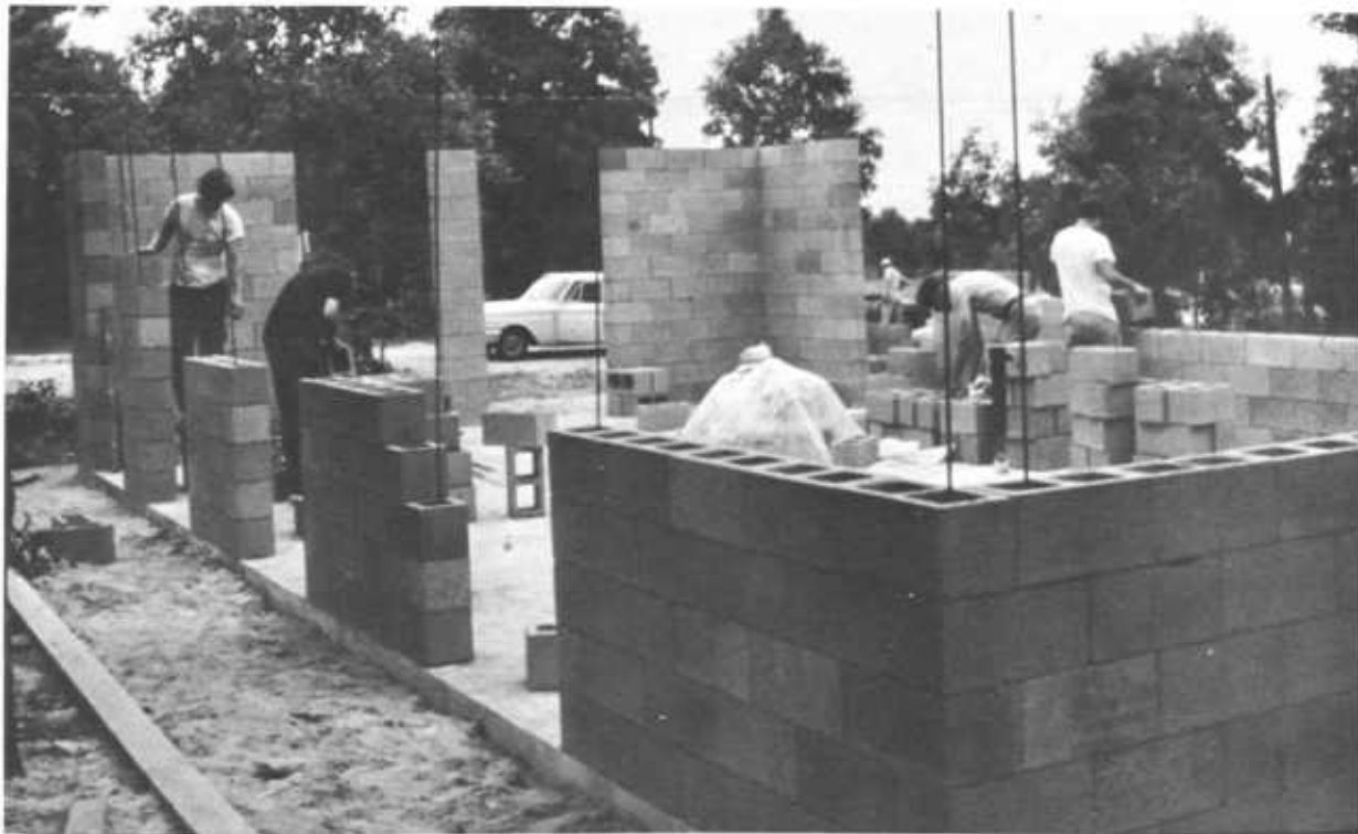
Dry stacking of concrete block walls at a self-help project in Gainesville, Florida.
