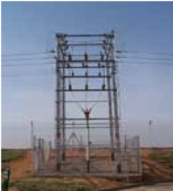
In Gujarat, separating the power cables carrying electricity to farmers from those supplying other rural users, such as domestic households and industries, had positive impacts much greater than anticipated. Photo Credit: Terry Clayton, IWMI.
