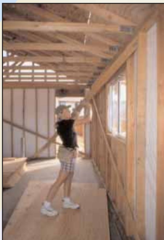
Under USDA's Mutual Self-Help Housing Program, rural people can become homeowners through an investment of "sweat equity." USDA Photo
