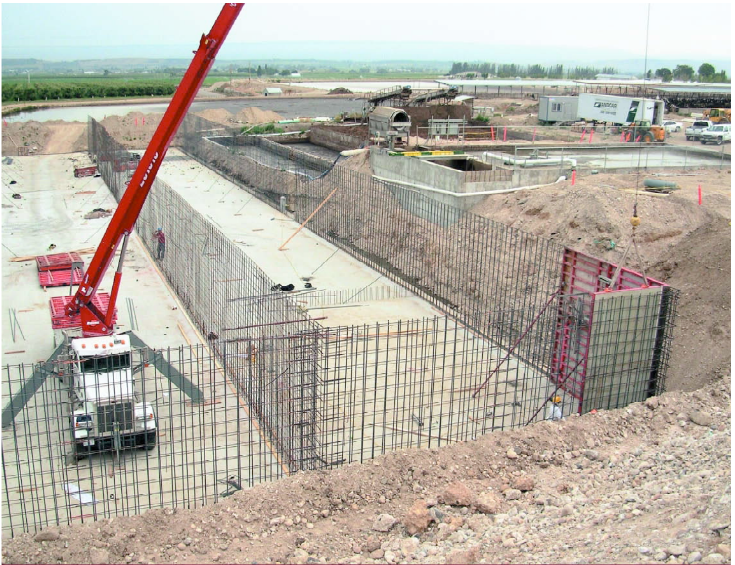
Forms are constructed to channel the flow of manure at the DeRuyter Dairy methane gas facility. Although this operation is not owned by a cooperative, this technology is well adapted for cooperatives to pursue.
