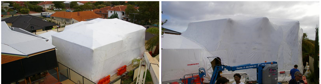
Figure 1. Khapra beetle infested house in Western Australia covered in shrink wrapped plastic sheeting in preparation for methyl bromide fumigation. Source: Under Raps Pty Ltd, n.d.
