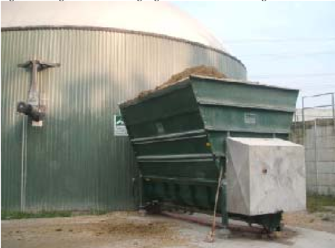
Figure 2.3: Organic material being augured into an anaerobic digester
