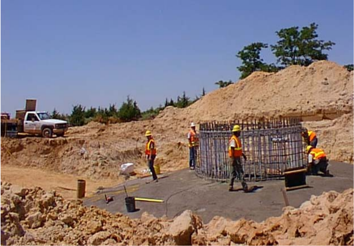
Photo 2. Constructing a wind turbine foundation in Woodward County, Oklahoma (Oklahoma Municipal Power Authority 2003)
