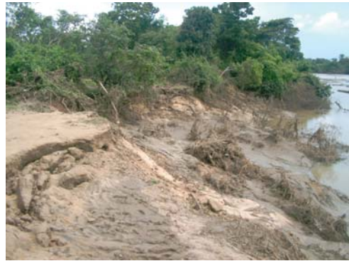
Example of a damaged river bank.
